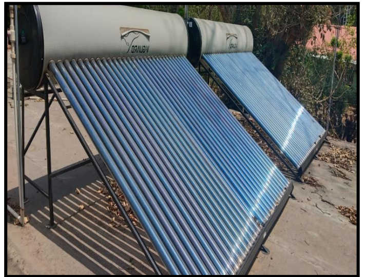
HOT WATER SOLAR PANEL
